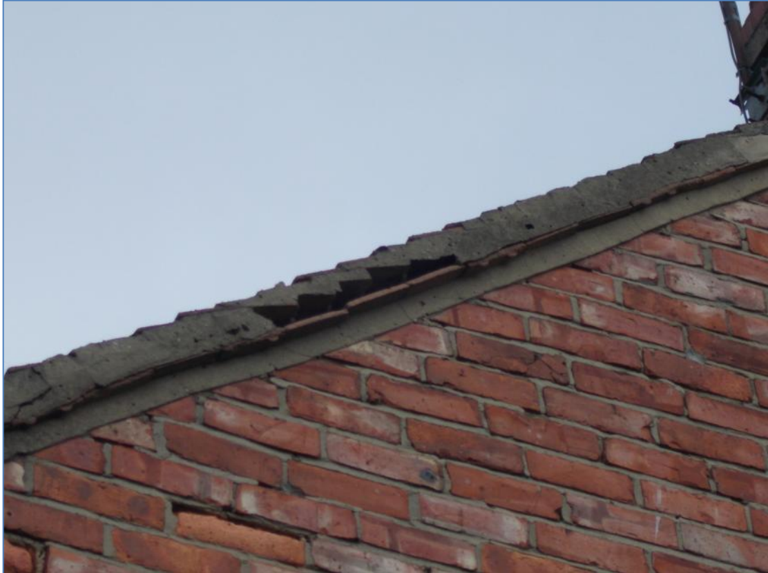
Photograph 3 - Section of absent mortar on south-west elevation.
